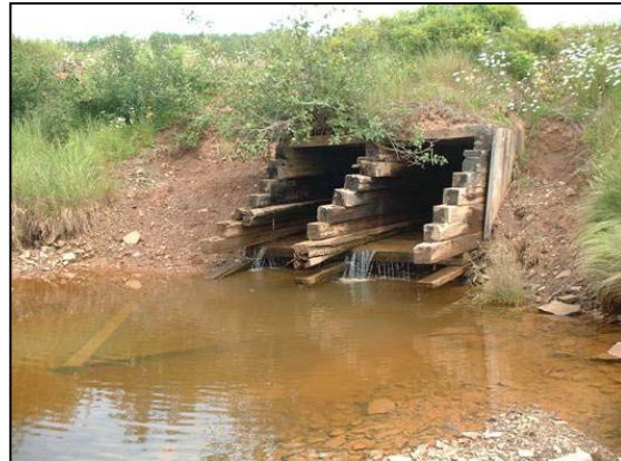
Figure 25. Downstream view of the culvert that has not been placed flush to the creek bottom.
