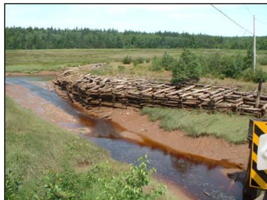
Figure 18. Old wooden structure downstream of the bridge, possibly an old wharf. DU bank impoundment off to the right under the bridge.
