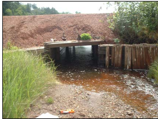
Figure 23. Upstream view of the culvert showing that the culvert is placed slightly off to one side with some pooling and slack water occurring to the sides of the culvert.
