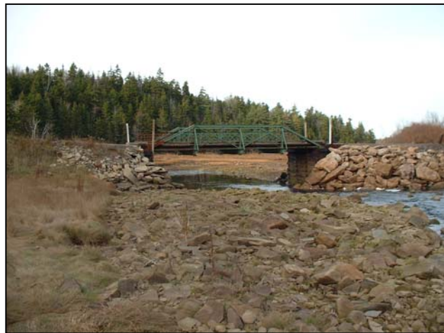
Figure 16. Downstream of the bridge clearly showing the build up of the banks with boulders.
