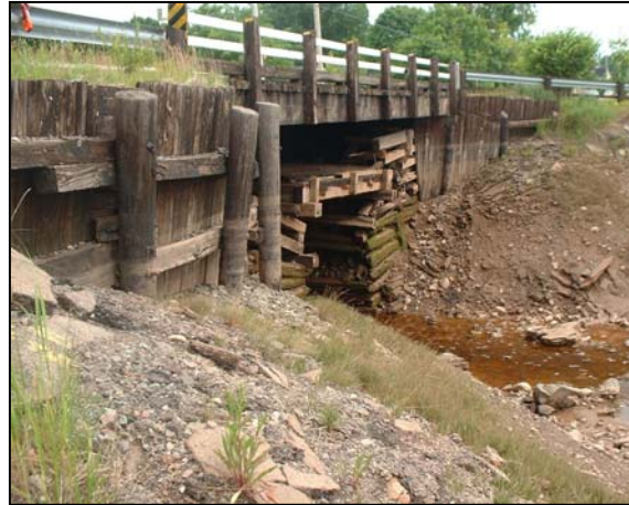
Figure 26. Downstream view of the bridge with the old structure visible under bridge.
