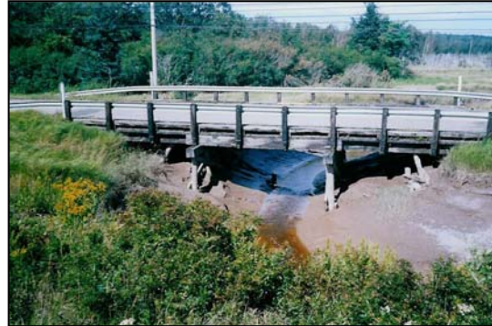
Figure 7. CCCB5B. Bridge seen from the downstream rail road. Salt marsh vegetation is visible on either side of the creek.
