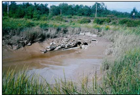
Figure 8. CCCB6C. Downstream of the rail crossing. The new, round, concrete culverts were punched through the old, square, wooden culverts. Photo taken at low tide.
