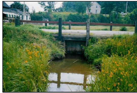
Figure 12. Downstream end of the crossing. The broken gate is visible. It is allowing some tidal flow, but should be removed to eliminate the small amount of pooling.
