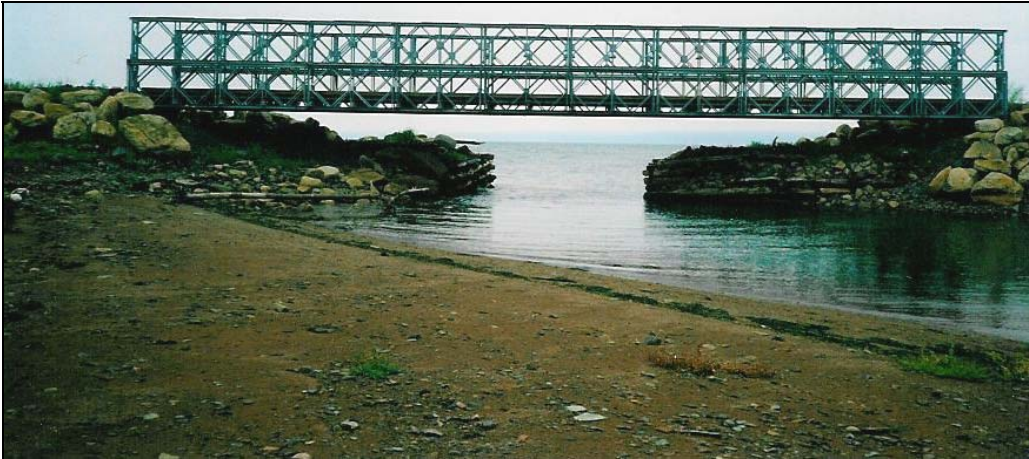
Figure 21. The bridge from the upstream beach (low tide) clearly showing the pinching of the river by the bank support structures.
