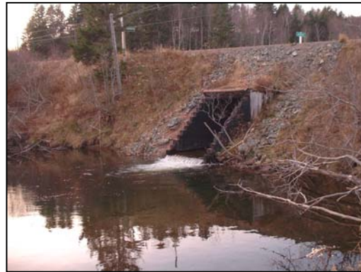
Figure 24. Downstream of crossing. The large pool in front of the culvert is visible as well as the high placement of the culvert.
