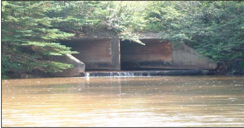
Left: culvert at high tide (3:45pm); water just barely reaches the underside of the base of the culvert. A small amount of freshwater continues to flow out of one side of the culvert.
