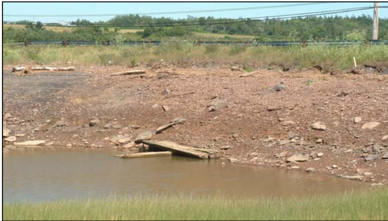
Left: downstream culvert three hours prior to high tide. Debris is present on banks and pooling of freshwater is occurring at the base of the culvert.
