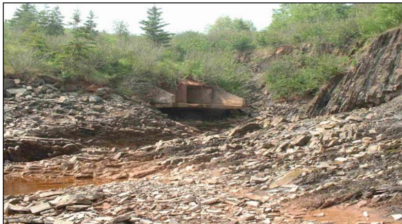
Left: downstream view of the culvert three hours before high tide. The water visible in the foreground to the left is the result of freshwater flow from under the roadbed.
