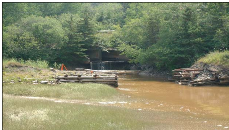
Right: culvert one hour prior to high tide, note the bridge remnants and small flooded salt marsh in the foreground.
