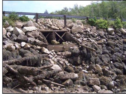
Figure 13. Downstream end of the culvert at low tide, filled with debris and in poor condition
