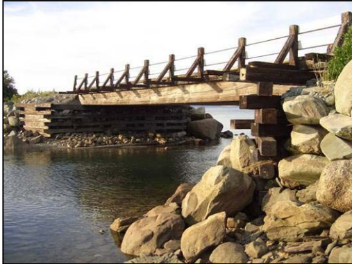
Figure 30. Upstream end of crossing, bridge is pinching the river channel.
