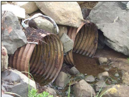
Figure 26. Downstream end of the culverts, rusted and collecting debris.
