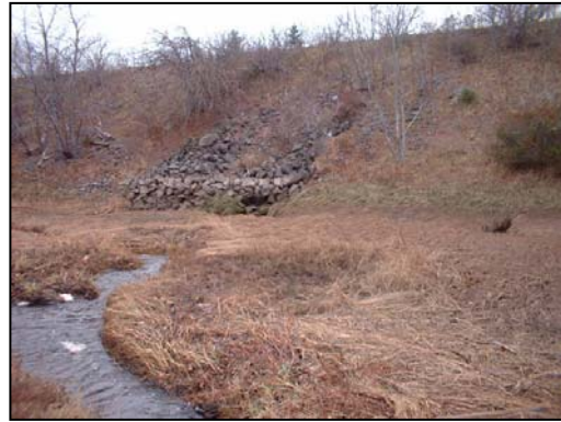
Figure 11. Upstream end of rail bed culverts, completely blocked by rock (DC6C)
