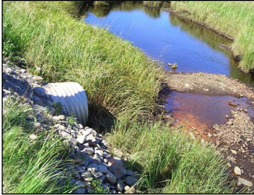
Figure 33. Downstream end of DC32C, undersized for the size of the system.
